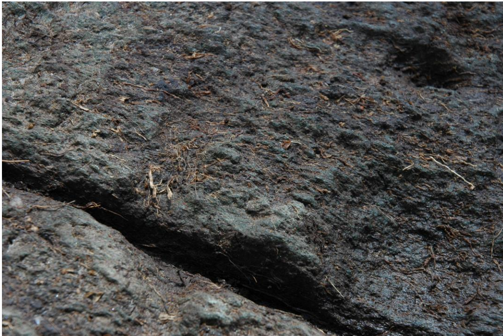
Root damage to rock surface
